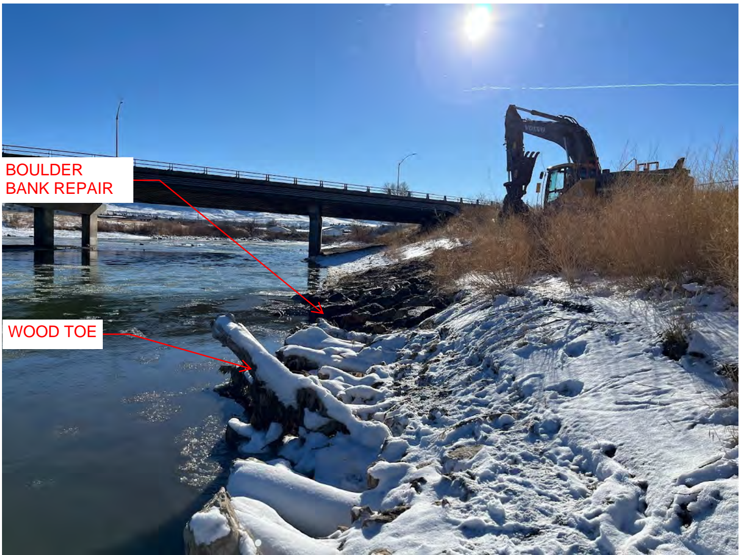
Figure 4: Image is taken on river left looking upstream. Finished product displaying the transition of the upstream bank into the wood toe.
