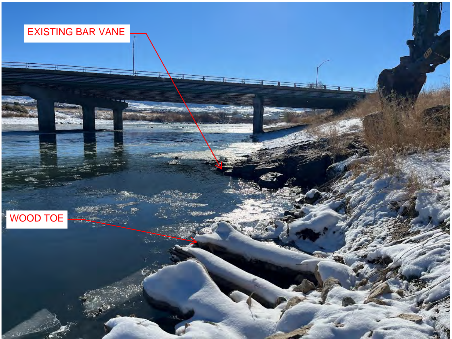
Figure 2: Prior to repair work. Image is taken on river left looking upstream. Erosion on bank can be seen between the existing bar vane and wood toe structures.
