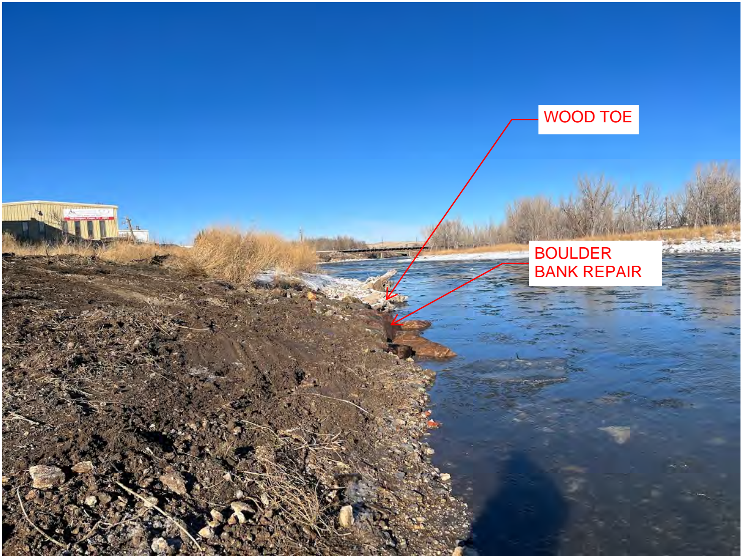
Figure 6: Image is taken on river left looking downstream. Finished product displaying the transition of the upstream bank into the wood toe.
