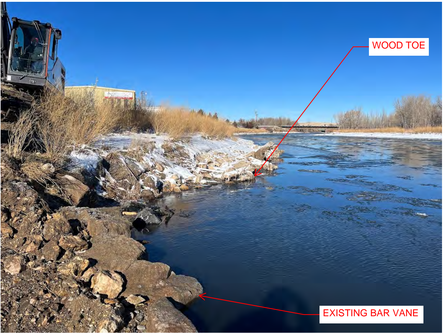
Figure 1: Prior to repair work. Image is taken on river left looking downstream. Erosion on bank can be seen between the existing bar vane and wood toe structures.
