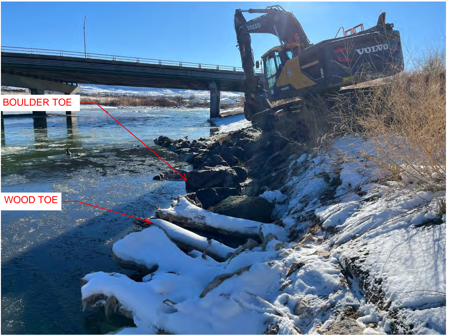
Figure 3: Image is taken on river left looking upstream. Setting boulder toe along area of bank erosion.
